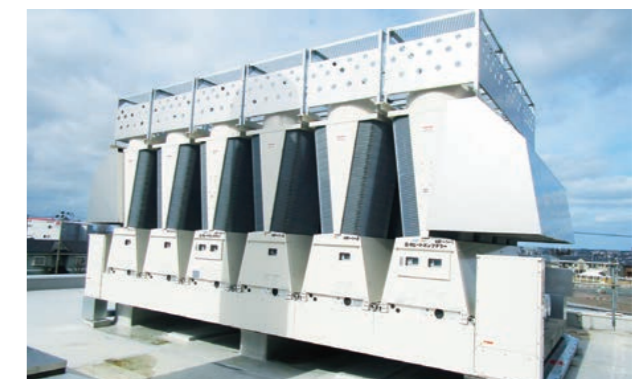
Air-cooled heat pump chiller introduced as part of our ESCO service (heat source equipment for ventilation)
