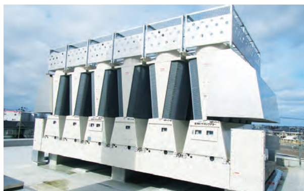
Air-cooled heat pump chiller introduced as part of our ESCO service (heat source equipment for ventilation)
