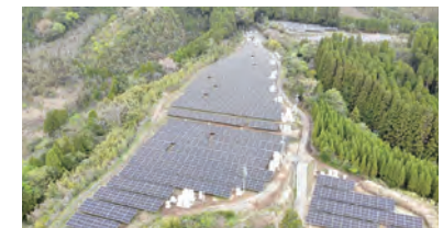
On-site photograph of storage battery facilities equipped with renewable energy facilities (Kagoshima Prefecture)
